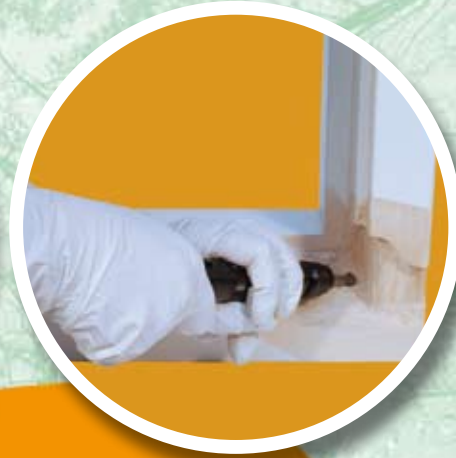
2. Remove all decay
